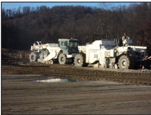
High production of lime drying and cement stabilization was easily achieved with multiple spreaders and mixers from Mt. Carmel's vast equipment fleet.
