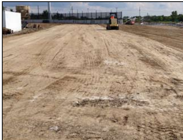
The lime modified subgrade has been completed in this area. What was rutting up to 3' deep is now stable and stiff.
