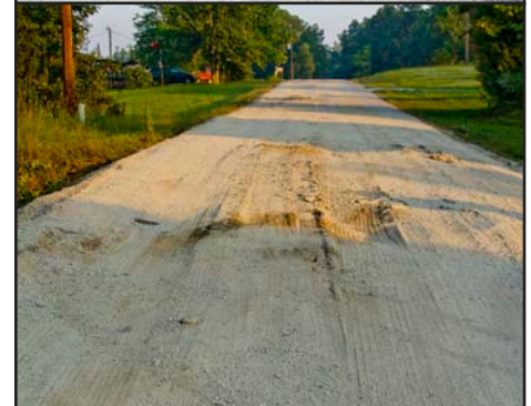
Photos from the roadway show the full extent of the damage. Maintenance crews attempted fill in the deep ruts with gravel but the source of the problem was deep beneath the roadway.
