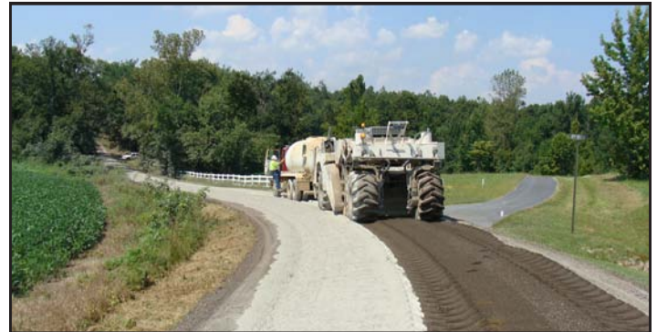
After cement application the section is remixed with water added in the machine's mixing drum to hydrate the cement and obtain the optimum moisture content for compaction.
