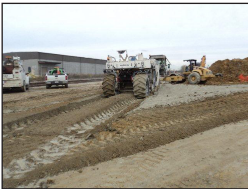
Mt. Carmel Stabilization Group utilized a Wirtgen WR 2400 for work on this project. With 25 similar Wirtgen mixers in it's fleet, Mt. Carmel can tailor production to meet any project demand.
