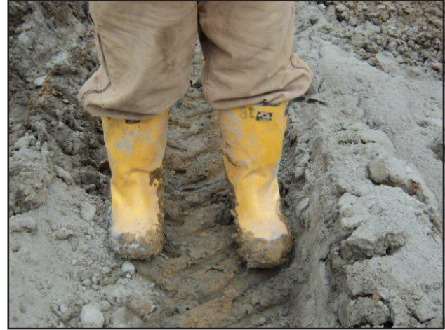
With high moisture contents throughout the site, severe rutting was common prior to cement stabilization.
